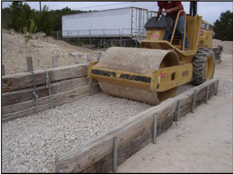
LIFTING PLATES POSITIONED BETWEEN TIES AND COVERED WITH FIRST LIFT OF COMPACTED SOIL/AGGREGATE
