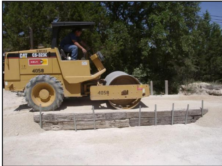
COVER SOIL/AGGREGATE IS UNIFORMLY SPREAD AND COMPACTED USING FIELD-SCALE EQUIPMENT AND PROCEDURES
