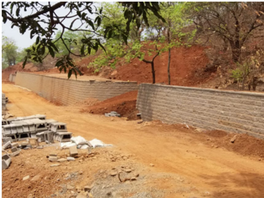
Project in India for retaining walls undertaken by Prayosa (Allan Block Licensee)
