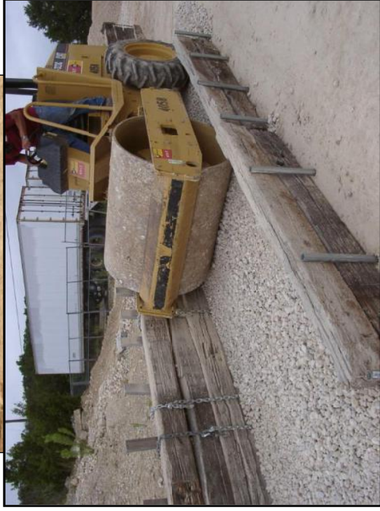
LIFTING PLATES POSITIONED BETWEEN TIES AND COVERED WITH FIRST LIFT OF COMPACTED SOIL/AGGREGATE
