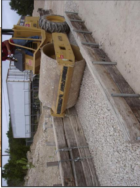
LIFTING PLATES POSITIONED BETWEEN TIES AND COVERED WITH FIRST LIFT OF COMPACTED SOIL/AGGREGATE
