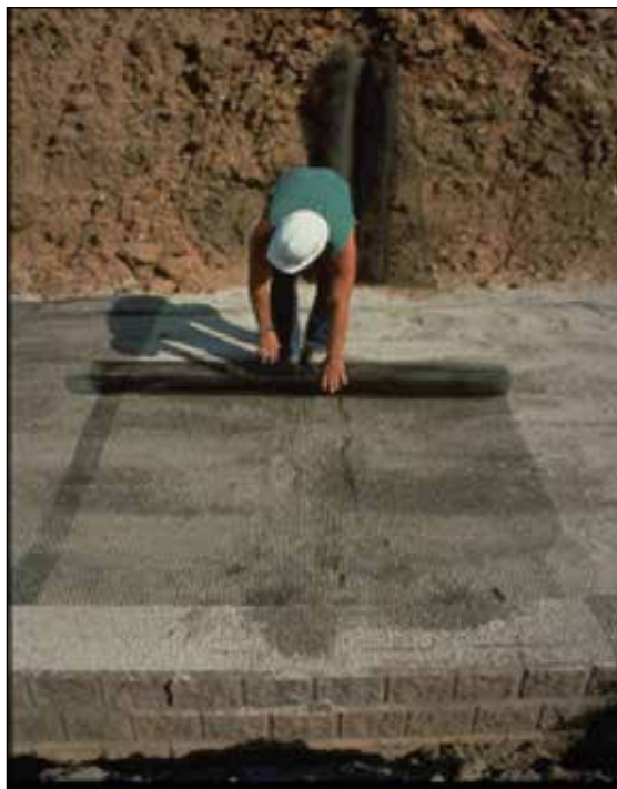
Figure 7. Improperly Placed Geogrid (geogrid is being overlapped at the face and without soil between geogrid sheets)
