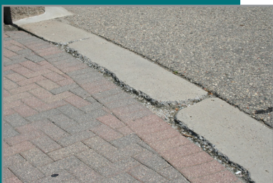
FIGURE 3 BURNSVILLE, MN BUS TERMINAL, CONCRETE DEGRADATION (2012)
