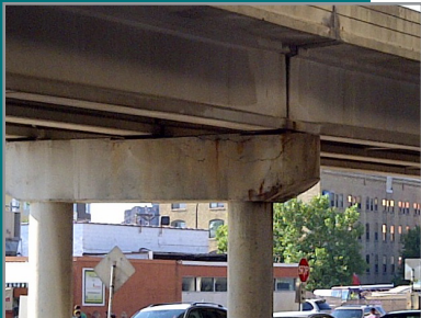
FIGURE 2 MN I35 BRIDGE PIER DAMAGE (2012)
