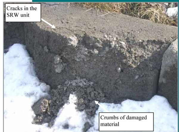
FIGURE 4 FREEZE-THAW DAMAGE ON SRW UNIT IN THE FIELD (REF. 6., FIGURE 49)
