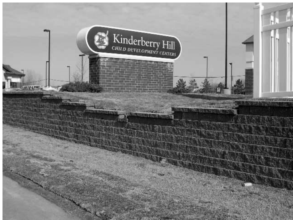
Figure 11-1: Surface Drainage Feature on a SRW
